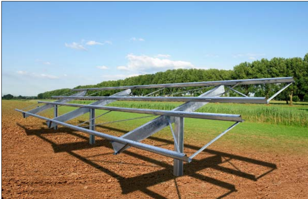
Plate 2.1: Example of a solar PV support structure
